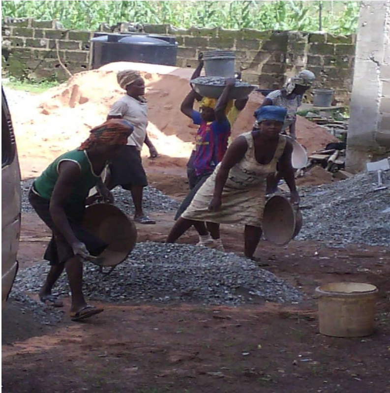
Figure 2: Women Laborers in the job of Concrete Mixing in an ongoing building construction in Abakaliki. Photo taken by the author during field work on 10/30/2019
