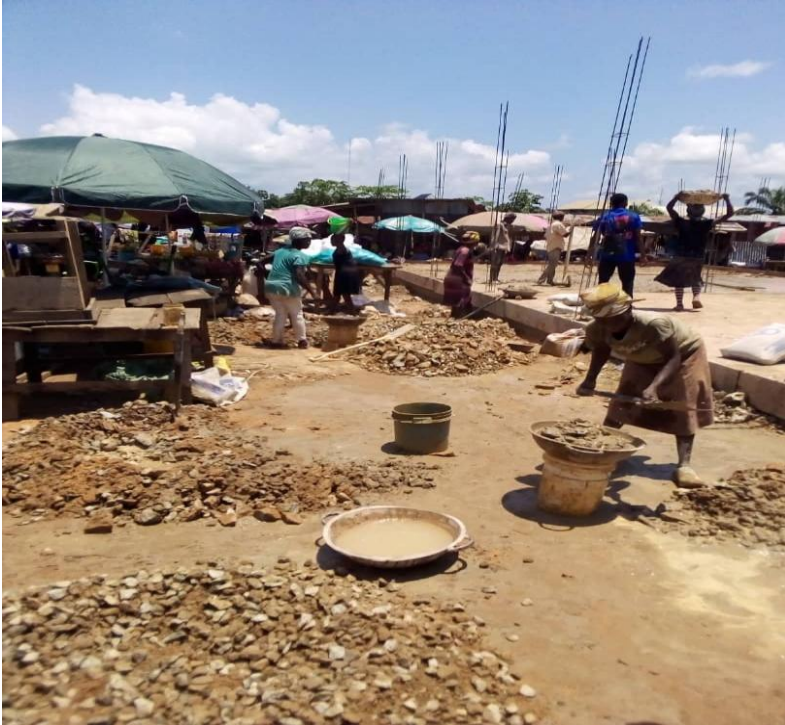
Figure 5: Women Laborers mixing concrete in an ongoing construction of the New KpiriKpiri Ultra-Modern Market, Abakaliki. Photo taken by the author during field work on 09/07/2020
